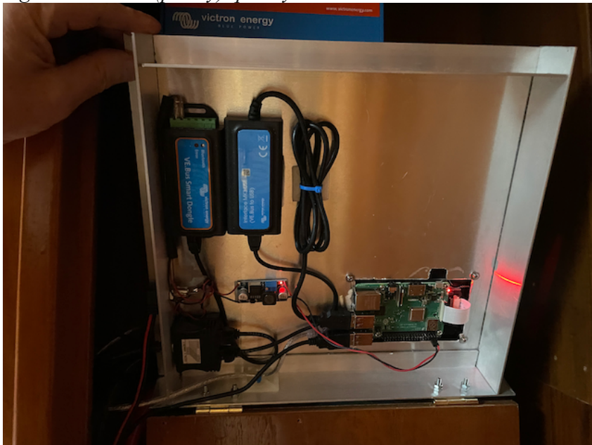
inside of aluminium box with electronics for data exchange
