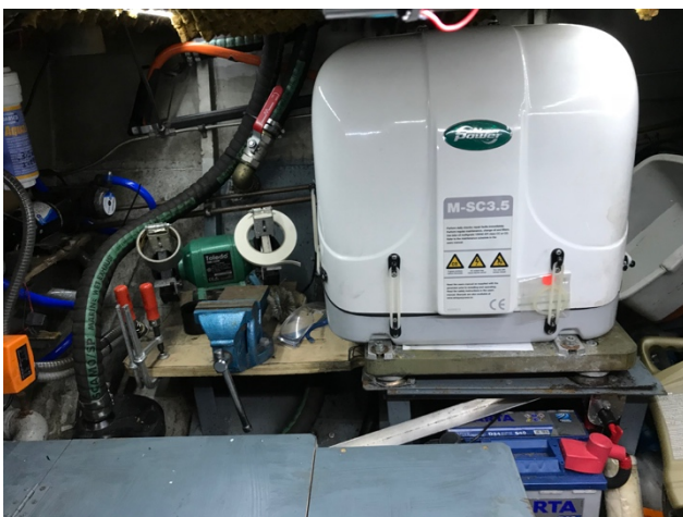
Whisper Generator 3.5 KVA
